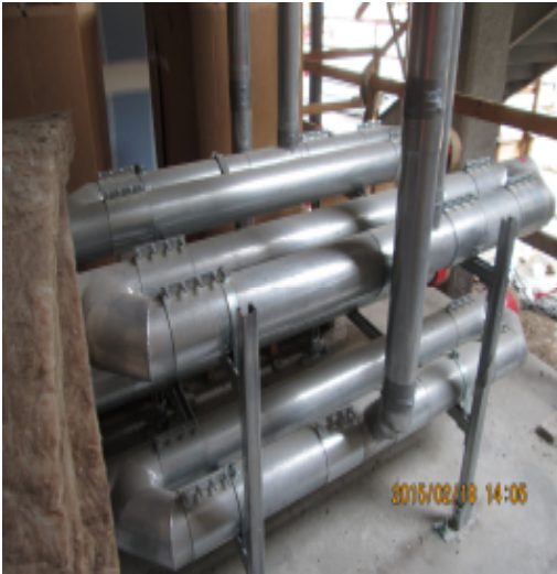
Pneumatic Tube Connection To Blowers
