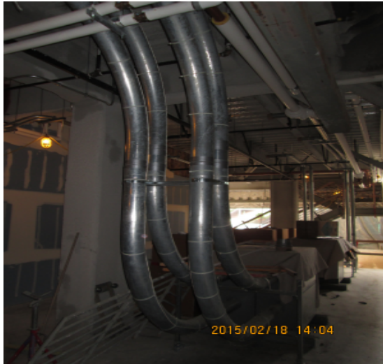
Pneumatic Tube transition to floor mounted diverters
