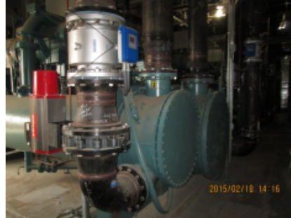
Chiller Piping Metering
